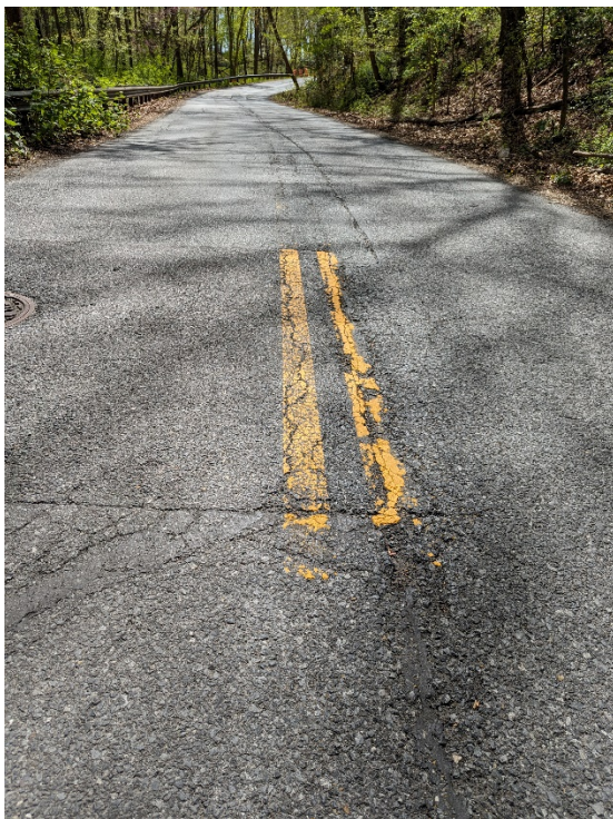
Yellow Striping not continuous
